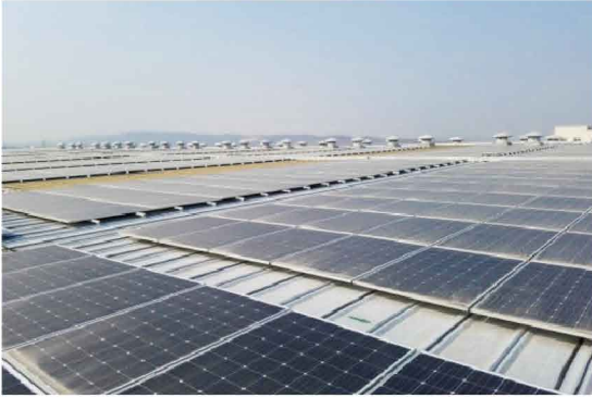
光伏太阳能支架 Photovoltaic solar mounting system
